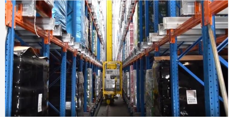
Automated Racking Systems
